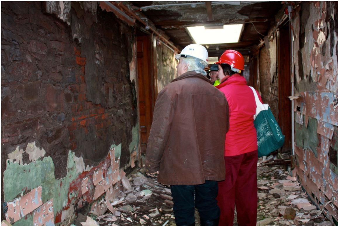
The result of a recent wall collapse in December 2012.
